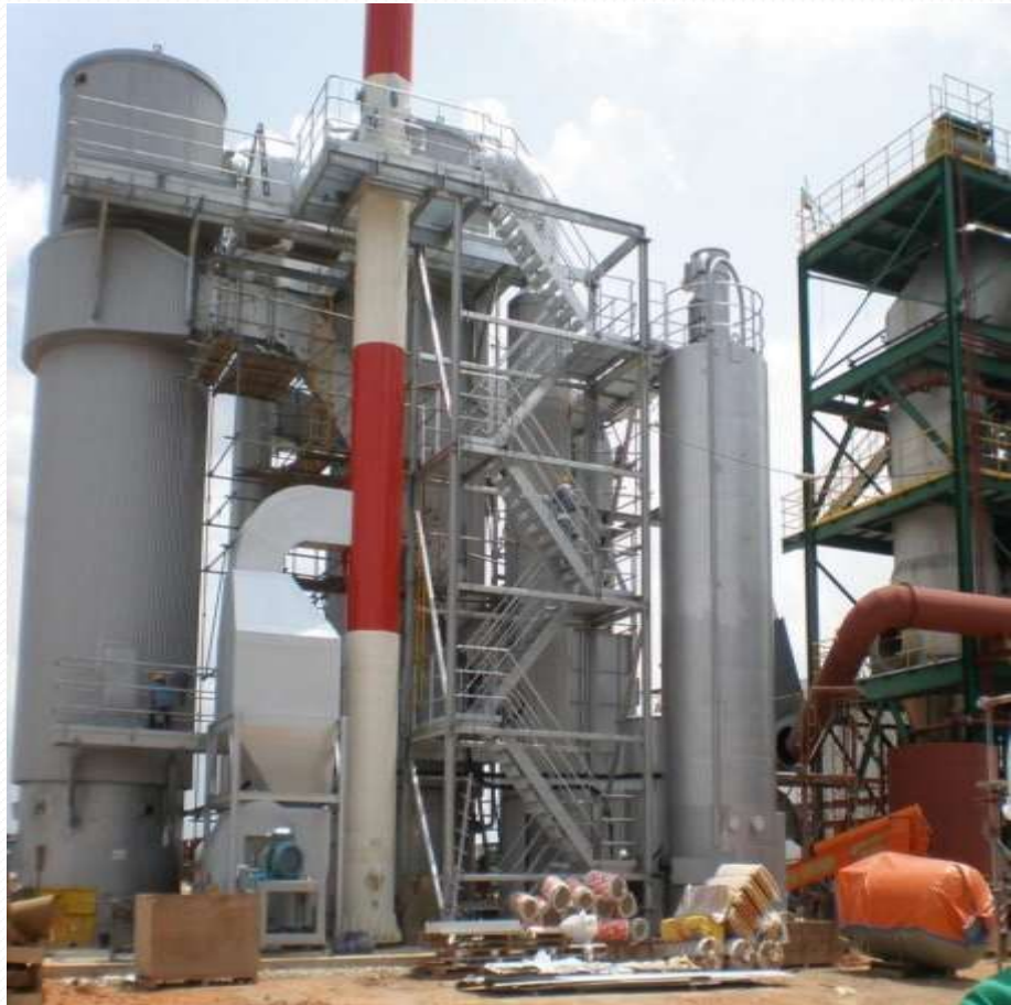
Scheduled Waste Incinerator
